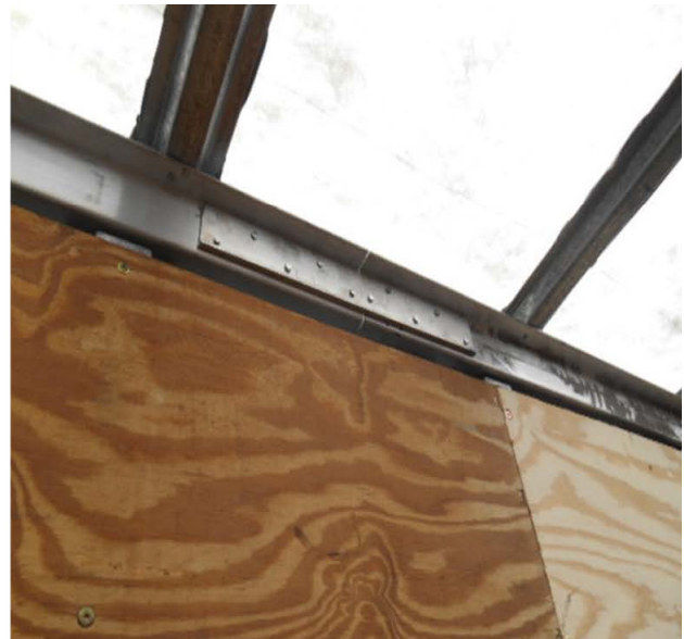
Fig. 2.26 Top rail improper repair—splice plate does not span two posts
