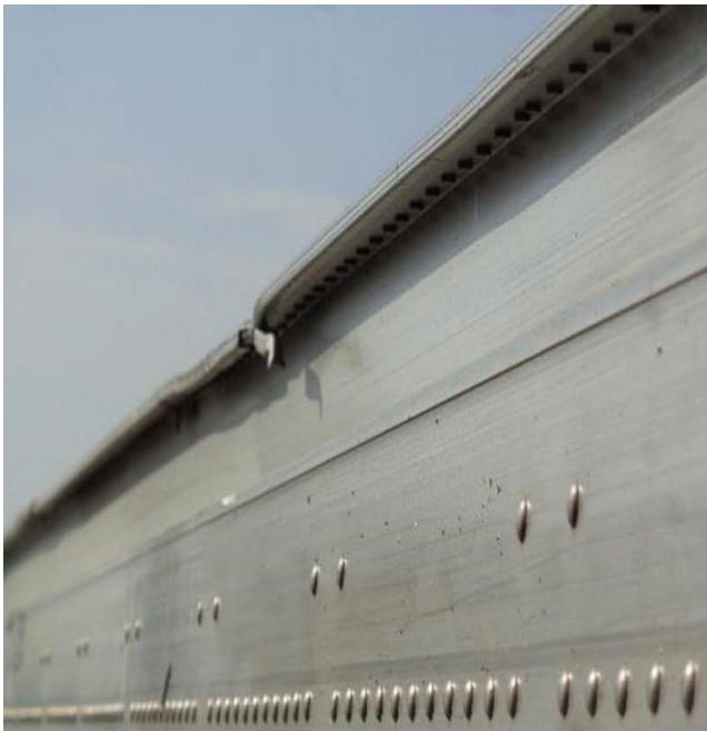
Fig. 2.21 Top rail broken
