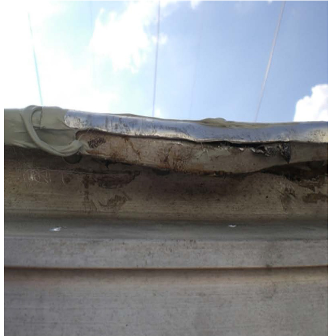
Fig. 2.20 Top rail crack
