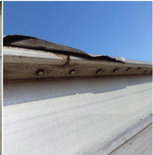
Fig. 2.22 Top rail broken
