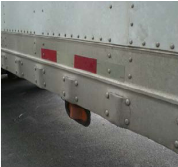
Fig. 2.6 Bottom rail deformation
