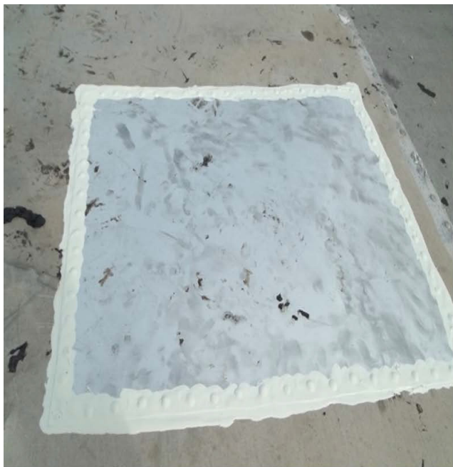
Fig. 2.35 Roof sheet patch exceeds 12 in. × 36 in.
