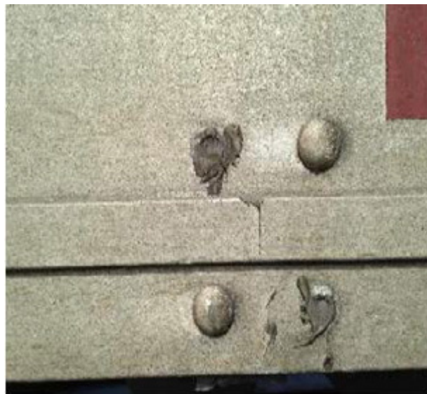
Fig. 2.11 Securement defect—broken rivets
