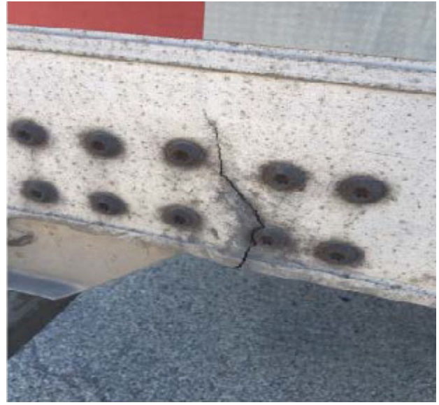
Fig. 2.5 Bottom rail crack
