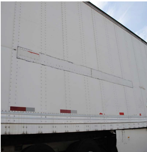
Fig. 2.33 Side panel improper repair
